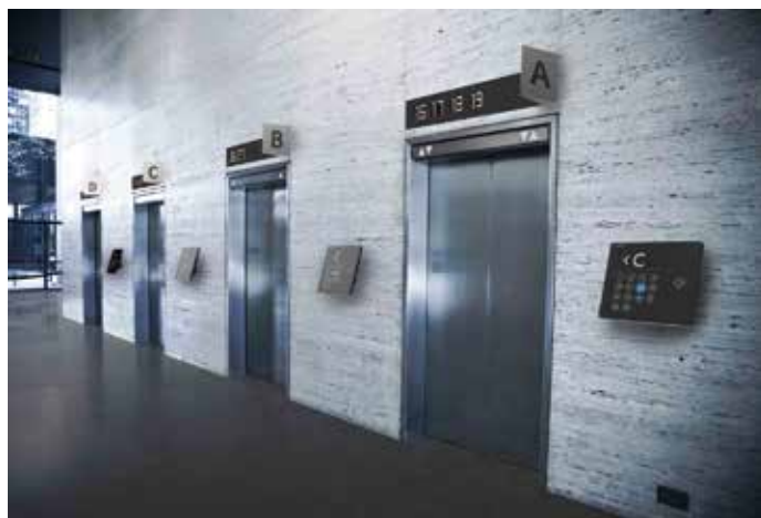
Toshiba's FLOORNAVI system sends users to the correct elevator.
