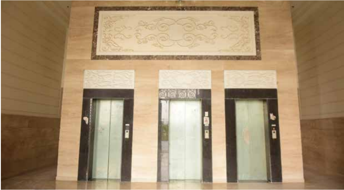
The development uses Toshiba high-speed elevators.
